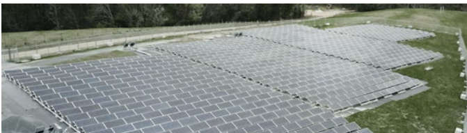
500 kW G20 System, GA
