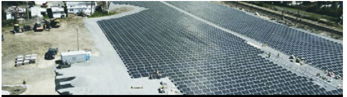
2.5 MW Ballasted Brownfield, NJ
